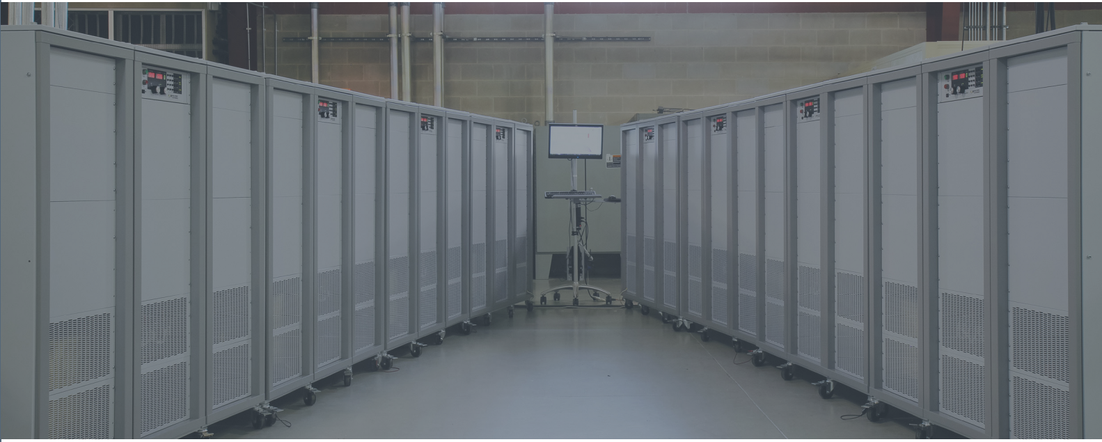
Qty (8) 250 kW MT Series units in master-slave parallel to form a 2 MW system
