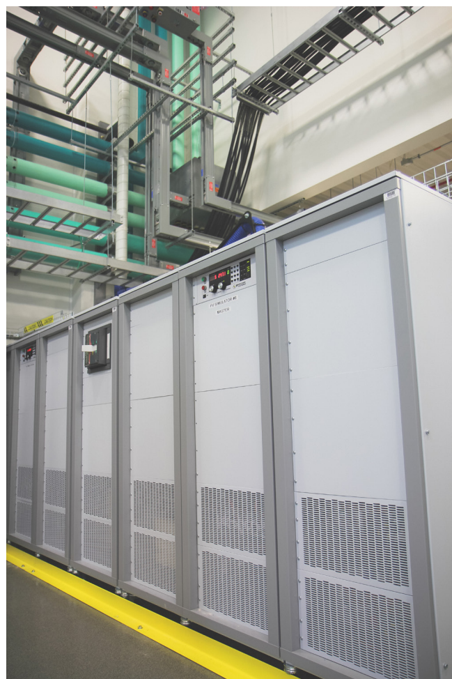
1.5 MW solar array emulator using Magna-Power MT Series power supplies at the National Renewable Energy Laboratory in Golden, Colorado USA
